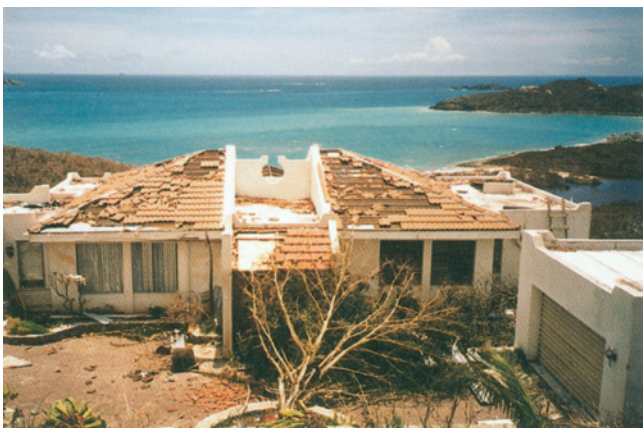
CS 16.11. After Hurricane Luis (front). High winds and flying debris responsible for downed trees, roof tile damage and solar water heater being ripped off. By David Morrison.
