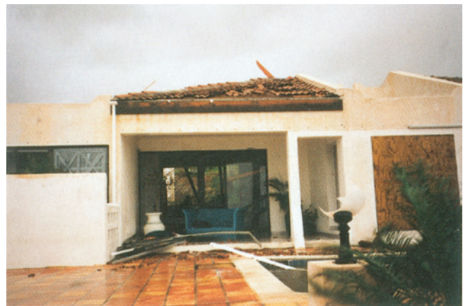
CS 16.10. After Hurricane Luis (back). Winds ripped off shutters and their tracks, while flying debris shattered clay tiles. By David Morrison.
