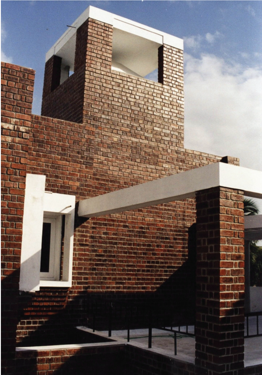
CS 5.1. Ventilation shaft.
