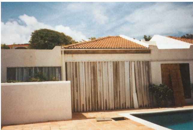
CS 16.9. Before Hurricane Luis, protected with aluminium shutters, by David Morrison.
